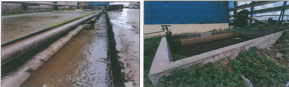
450 m 3 Collection tank and pumps arranged at the back of warehouse no. 3
