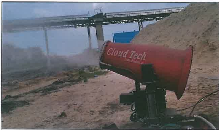
Fog Cannon installed at the Bagasse yard increasing the moisture in the area and reducing emissions.
