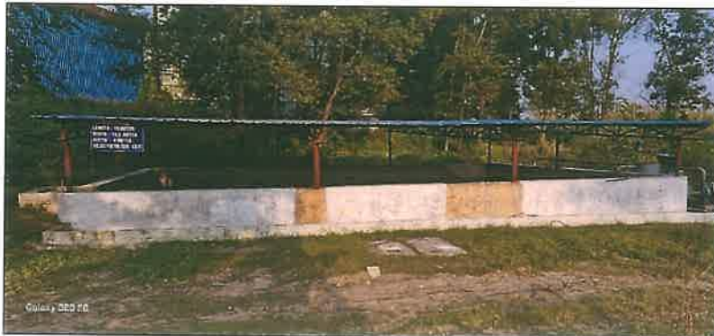
450 m 3 Capacity collection tank along with pumps arranged to collect Leachate.
