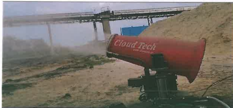
Fog Cannon installed at the Bagasse yard increasing the moisture in the area and reducing emissions.
